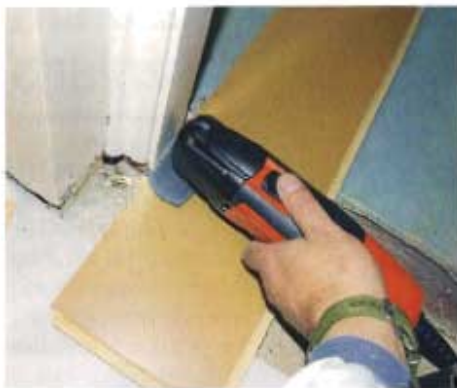
▲ Pic. 1 Using a sawing blade it's ideal for trimming door linings when fitting laminate
